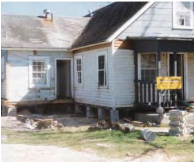
Figure 2. After decades of settling into the ground, this house (top) is showing serious moisture damage. New floor joists (middle) provide a sound structure for jacking. The framing nailed to the wall helps to pick up individual studs and the corner post. Note the new elevation of the porch rail relative to the concrete porch (bottom) as the house comes up.
