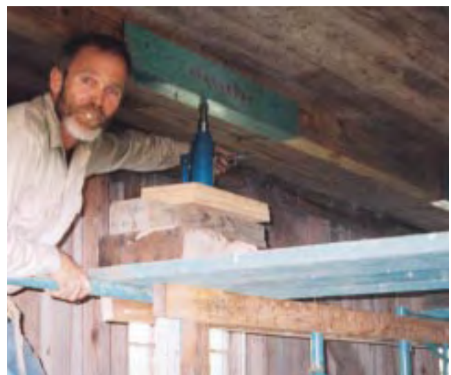
Figure 1. The author uses three types of jacks (from left in top photo): hydraulic, screw, and hypoid gear. Steel angle slips, predrilled for attaching with duplex nails, spread the load over a larger bearing surface (bottom photo).
