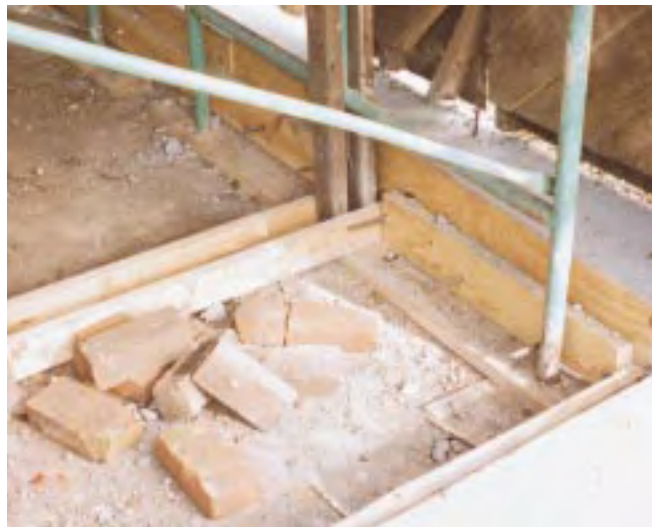
Figure 4. Staging made a convenient platform for jacking the carriage house (top), but it had to be thoroughly braced all the way to the ground. In addition to continuous cross-bracing in both directions, the author set 6x6 posts under the critical jacking points (middle), and made stable bases for the scaffold legs (bottom) by drilling holes in 2x6s.
