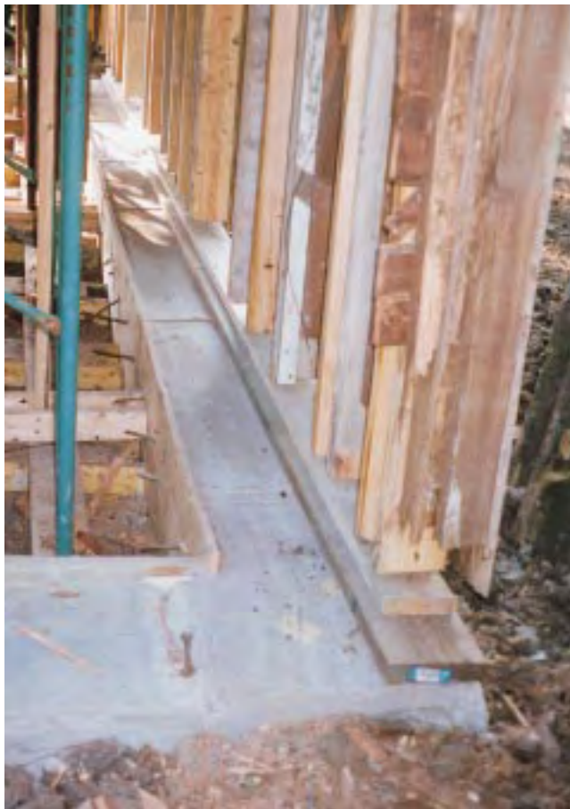
Figure 5. While the second story of the carriage house was suspended, the crew excavated, formed, and poured new footings (top), then repaired the wall framing and lowered the building onto new PT sills.
