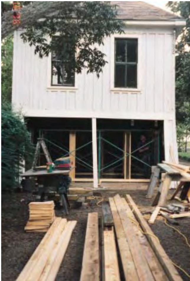
Figure 3. This turn-of-the-century carriage house was 19 inches out of level and 12 inches out of plumb before renovation. Termites had made mincemeat of much of its wall framing.
