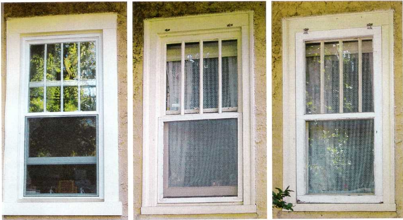
While the owner of this house spent extra money on this replacement window (left) for a custom muntin pattern to match the original, the stark white color, shallow muntin depth and lack of divided lites fail to convey the feel of the original (center). The trim around the replacement window was also capped with aluminum, another “no maintenance” effort that ruins the appearance of the window (notice the loss of the backband surrounding the trim). It will create a long-term problem when water trapped behind the aluminum rots the wood beneath. A level of thermal resistance comparable to that of a new window can be obtained by adding a storm window to the original (right).
