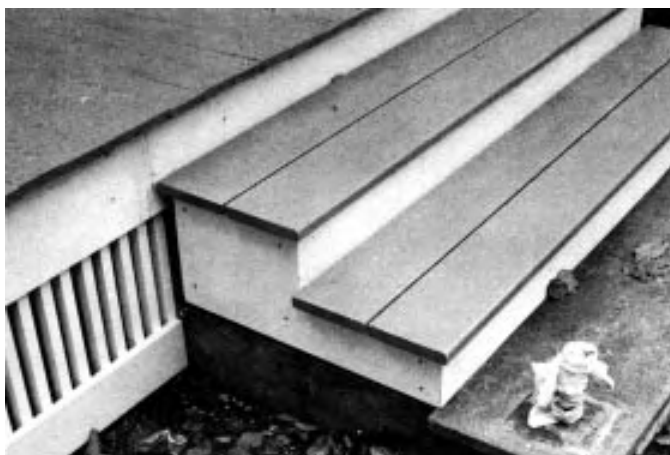
Figure 3. The finished steps fit in neatly with the rest of the porch — and will last.
