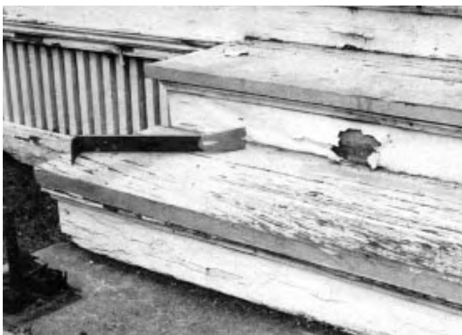
Figure 1. Paint peeling down to bare wood indicates excessive moisture in the woodwork. The buckling paint on the second riser is a result of decay.
