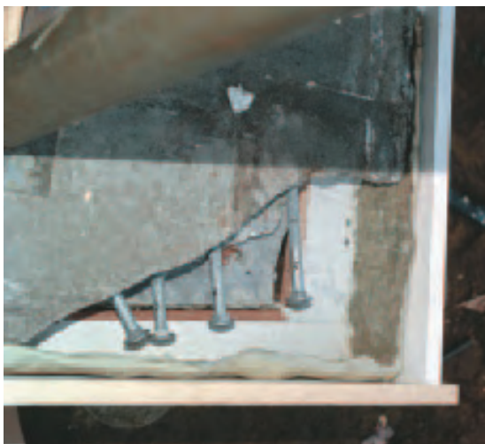
Figure 2. To repair a missing corner of the textured concrete floor, the crew first made a latex mold of the opposite corner. The mold was then used to line the small form, to capture the edge texture. Galvanized bolts were epoxied in place to strengthen the new corner.
