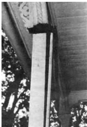
Figure 2. Columns wrapped in 1x stock conceal hidden damage. Take the columns apart very carefully because much of the material can be reused.
