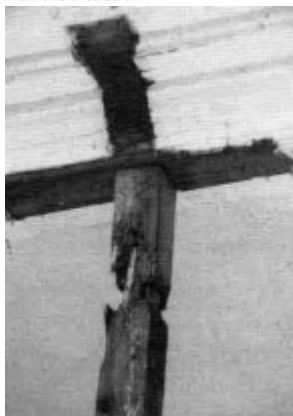
Figure 3. The post looks like it's been nibbled by beaver, but it's actually water damage.
