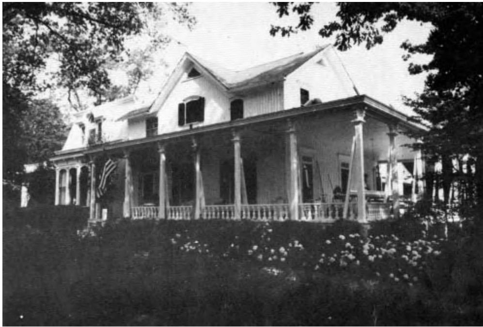
The wrap-around porch on this 1860s house had rotten joists, backed-up gutters, and decaying columns—a typical neglected porch.
