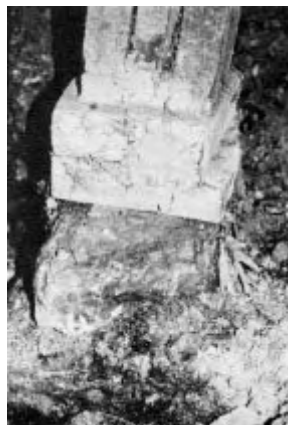
Figure 1. Dig down and you'll find surprises at footing level. This concrete footing, cracked apart, is resting on the original hunk of limestone.
