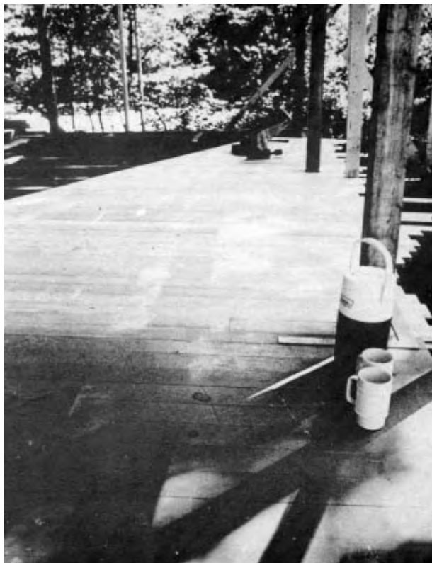
Figure 7. The thermos jug marks the spot where new tongue-and-groove porch flooring begins. Douglas fir flooring to match the old is still available.
