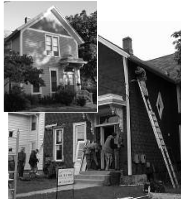
GPA’s Purchase/Rehab Program, instituted in 1987, turns problem properties back into architecturally appropriate historic homes that enhance the whole neighborhood and inspire other homeowners. Photos courtesy of GPA.
