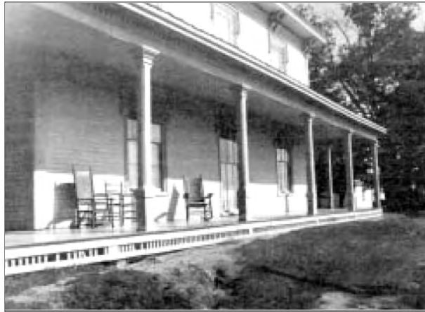
Figure 1. When built-in gutters were roofed over years ago, water flowed from the roof's edge, eroding the terrace.
